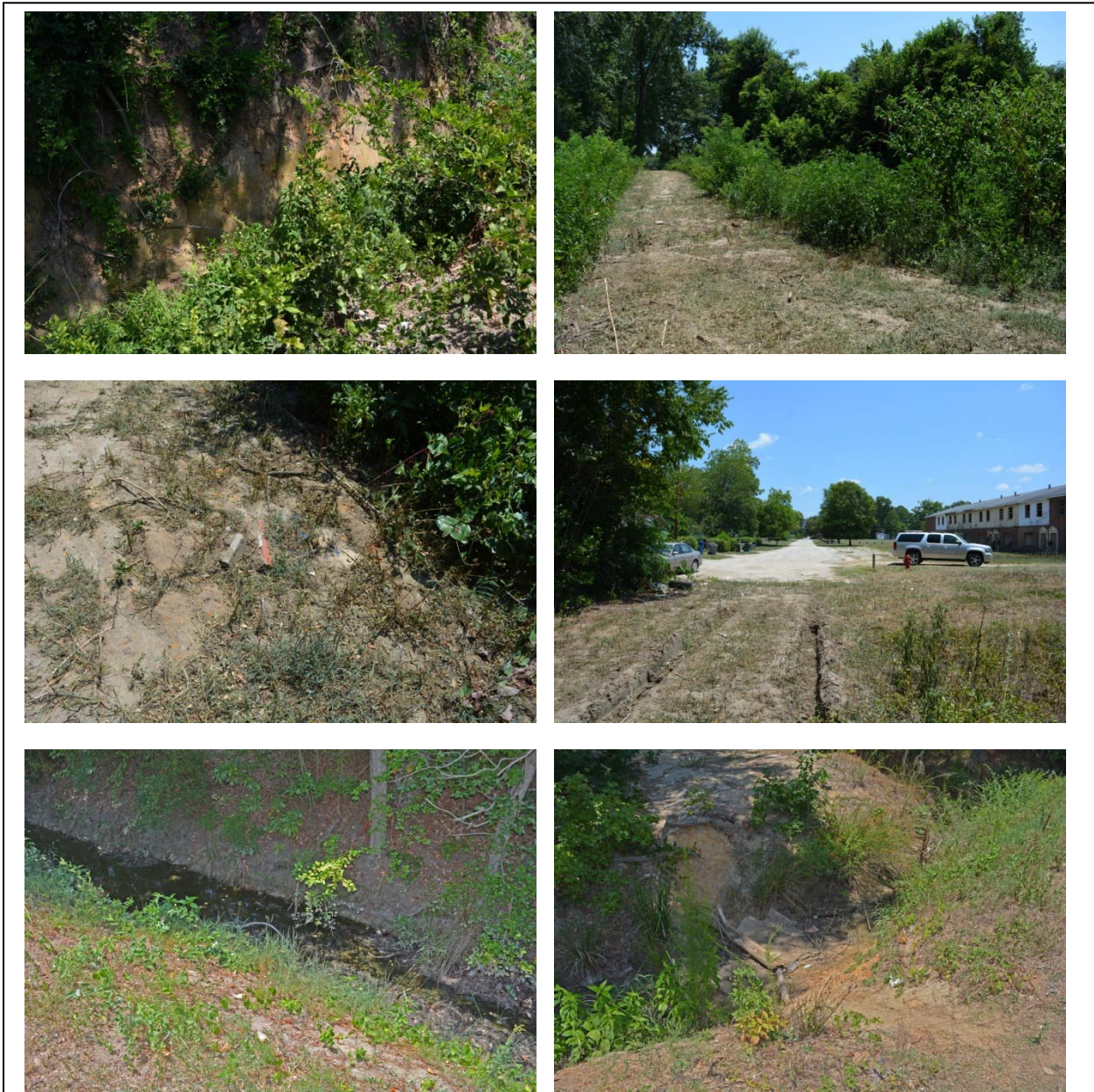
Figure 16. Ditches bordering the cemetery. Upper left photo shows the steep bank of the ditch along the north edge of the cemetery. Although recently cleaned, vegetation is already beginning to overtake the ditch from the north. Upper right photo shows the “easement” created where none exists. The cemetery is to the right of the photo. Middle left photo shows brick and stone in the “easement.” Middle right photo shows deep ruts created in the “easement” by the equipment needed to clean the ditch. Lower left photo shows stagnant water in the western ditch. Lower right photo shows a social trail through the ditch and trash that prevents water flow.
